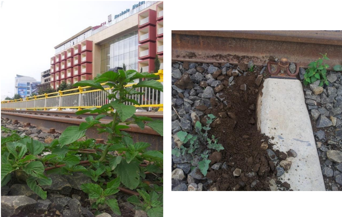
Figure 18: Ballast contamination and plant growth in front of Beshale hotel
