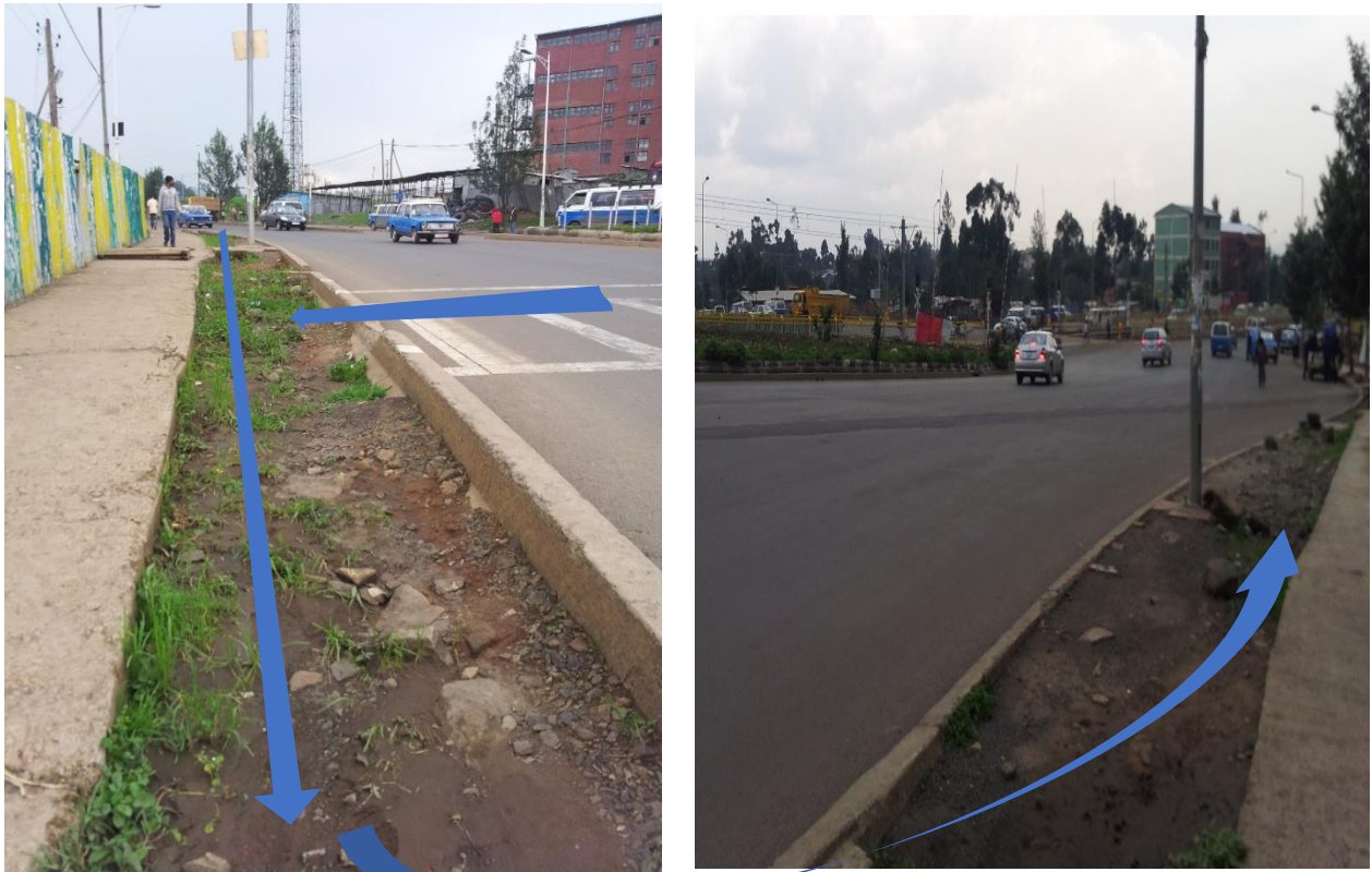
Figure 20: Surface flow pattern around Beshale Hotel
