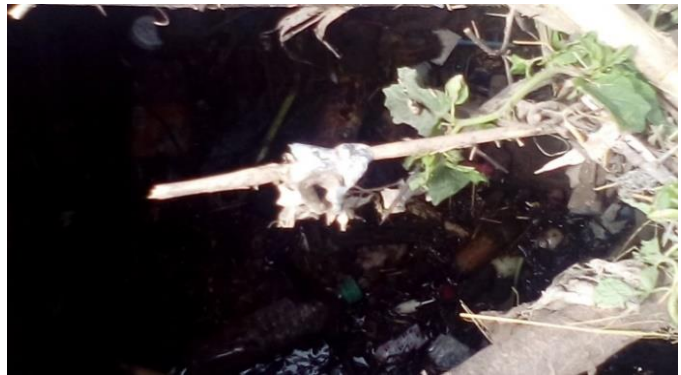
Figure 28: Blocked Sewerage due to alluvium secondary to Flooding, Akaki Kality Sub city, woreda 3, 2018
