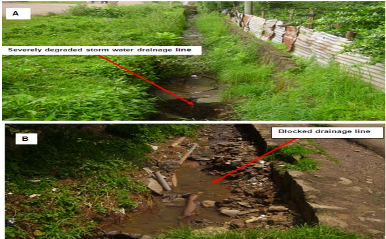
Fig-4.17 Severely degraded storm water drainage lines kebele 01/02(source: Field survey, 2009)
