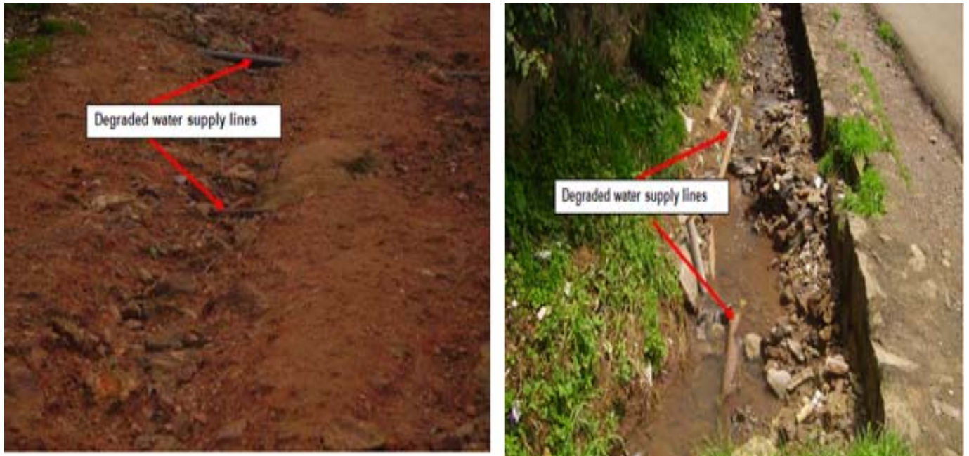
fig-4.20 Degraded water supply lines (source: Field survey, 2009).
