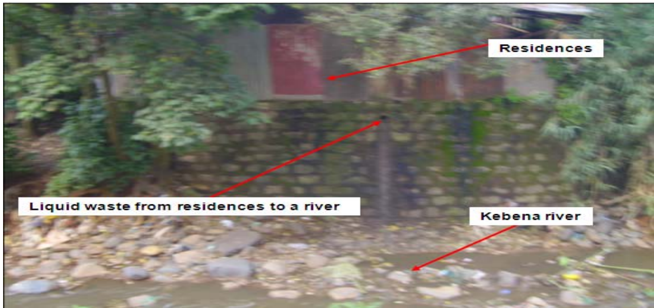
Fig.-4.14 Encroached river by illegal settlement kebele 08/15 (source: Field survey, 2009).
