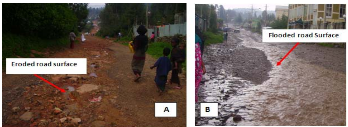
Fig-4.19 Highly eroded (A)and flooded road(B) surfaces (source: Field survey August, 2009).
