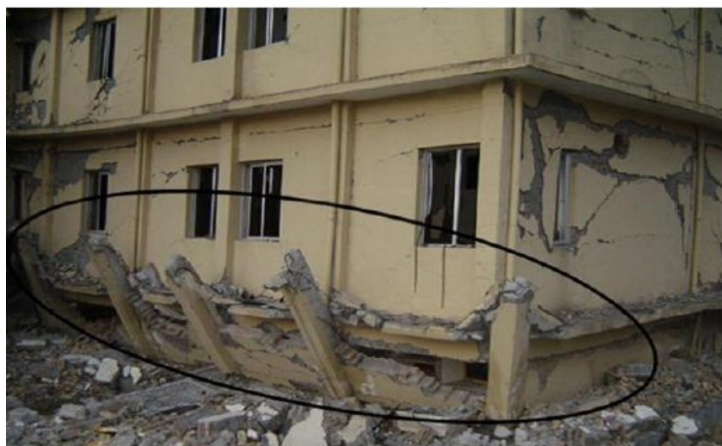
Figure 1-1- Shear Failure of Ground Story Columns
