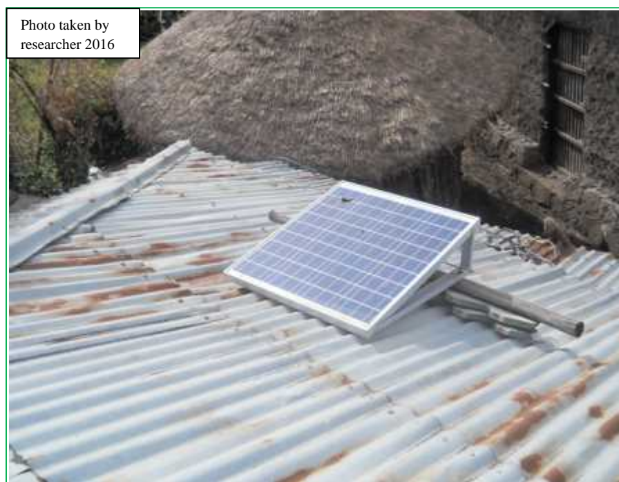
Figure 4.10 Support structures used is not strong.
