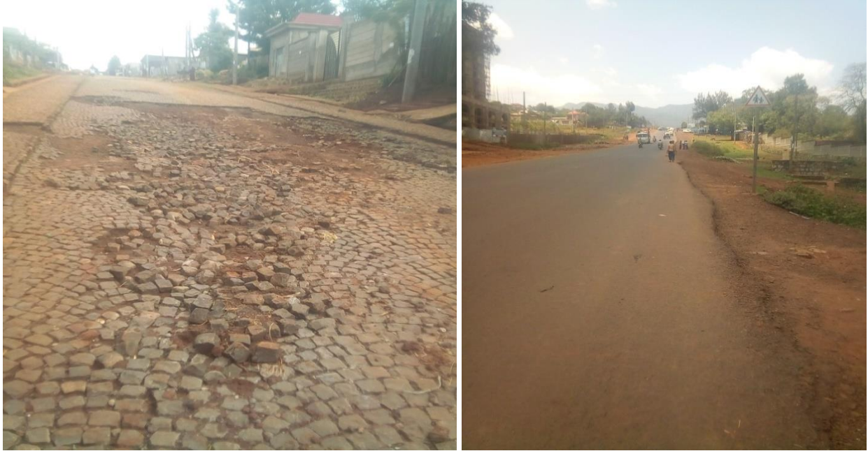
Fig. 4.4 poor road construction
