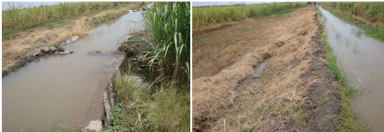
b) Overtopping and leakage problems on tertiary canals
