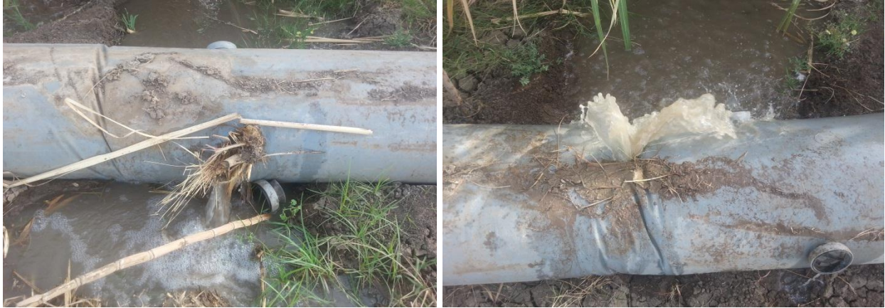
c) Torched and tired hydroflumes letting unwanted irrigation water to a field.
