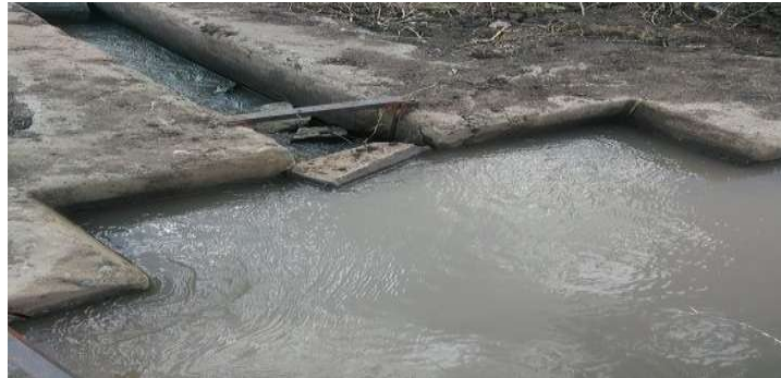
Figure 4.19 Malfunctioned main canal water distributing structure
