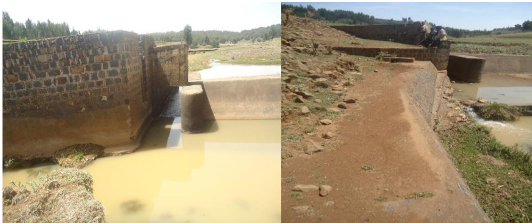
Figure 4.8 Damage on intake gate and under sluice Ydogite schemes
