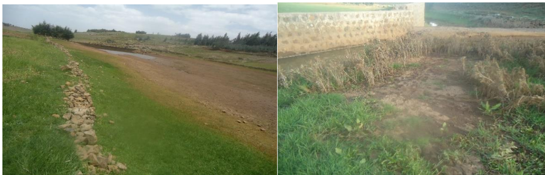
Figure 4.3 Silted-up head work structure Kendbersha and Fiadiangoa_1 schemes
