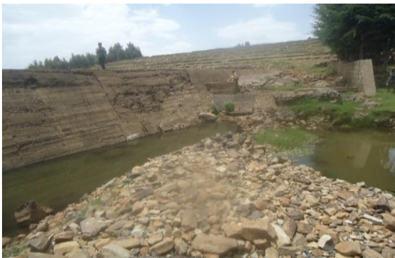
Figure 4.5 Downstream scoring Kendbersha irrigation scheme
