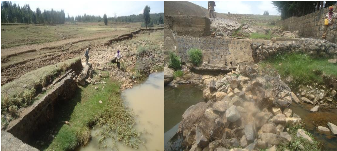
Figure 4.9 Damage on main canal Ydogite and Kendbersha
