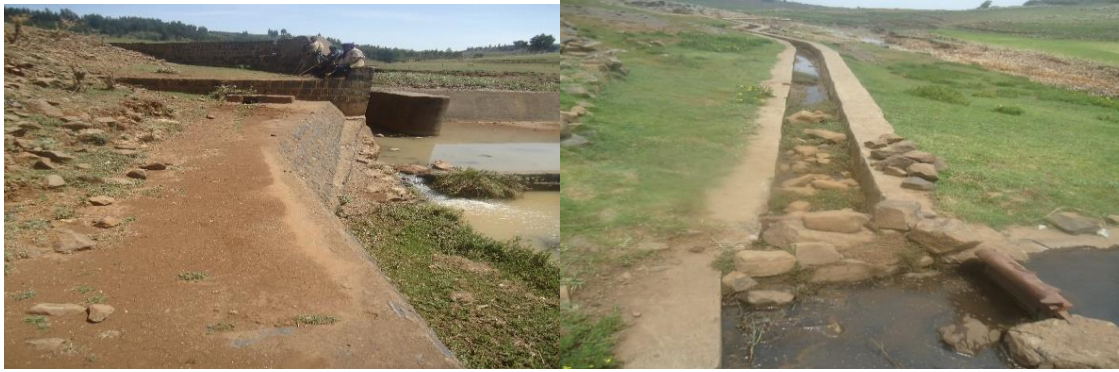
Figure 4.4 Silted-up canals Ydogite and Kendbersha irrigation schemes
