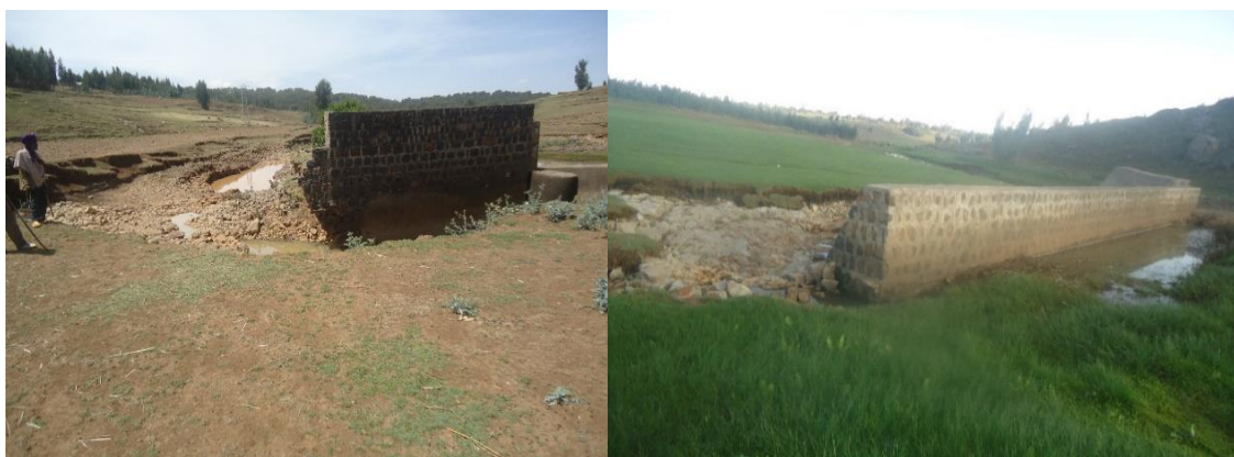
Figure 4.6 Damage on the retaining wall of Fiadiangoa_2 and Ydogite schemes
