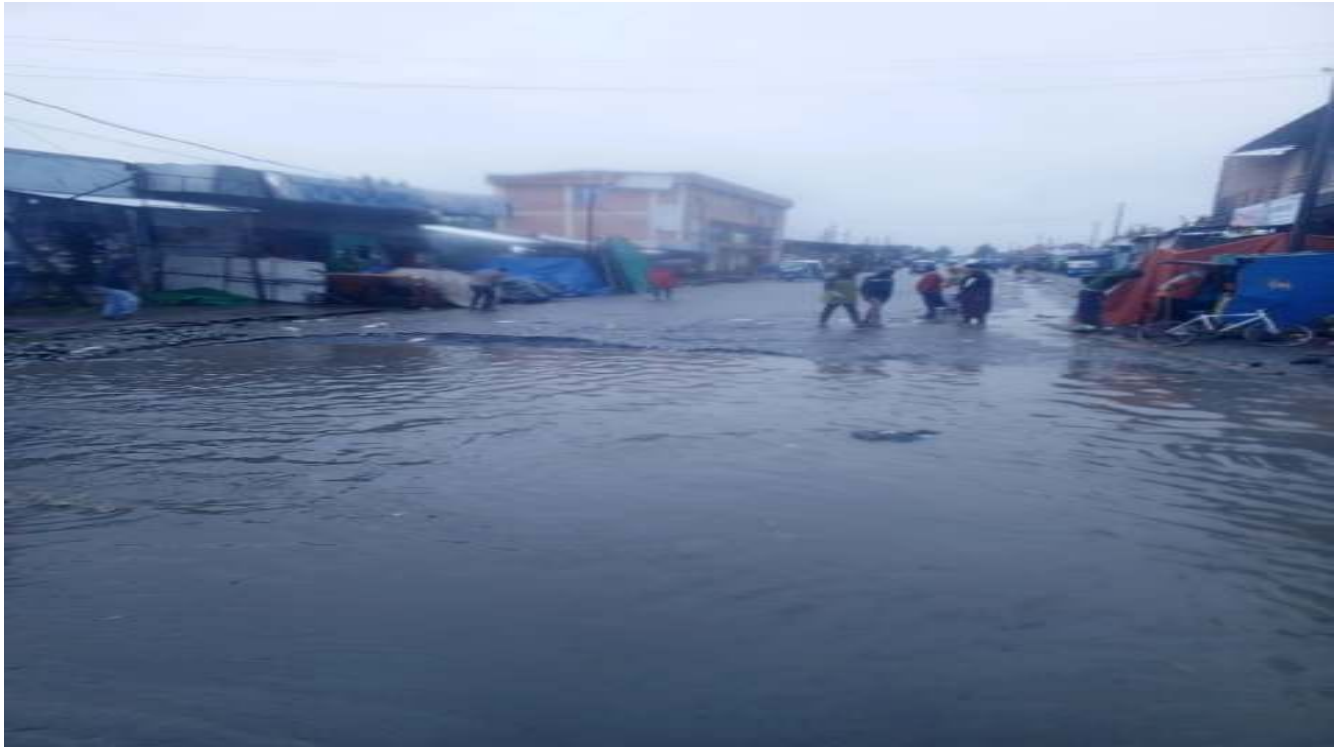
Photographs of below standard quality road infrastructure services
